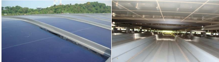
Figure 6- PV systems under monitoring on metal roof.
