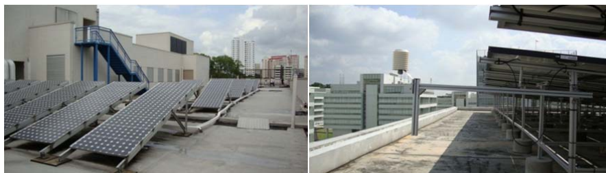
Figure 7- PV systems under monitoring on concrete rooftops.
