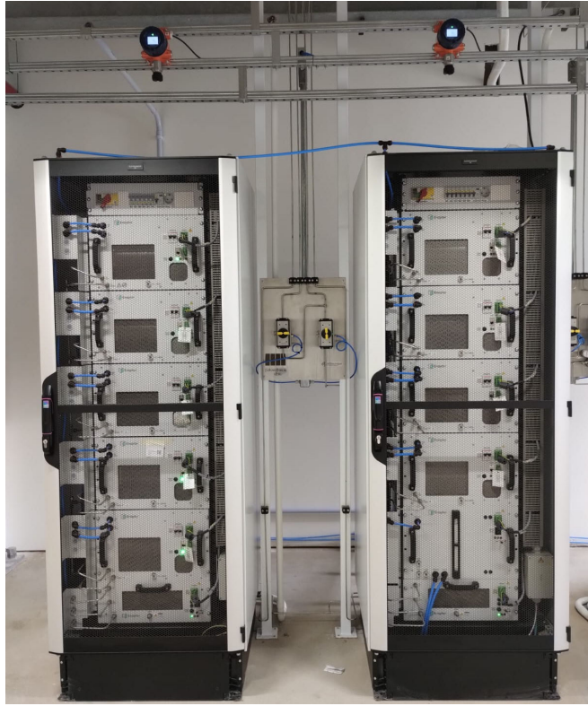
Figure 4 - Electrolyzer System at the Solar Energy Laboratory Fotovoltaica/UFSC in Florianópolis, Brazil.
