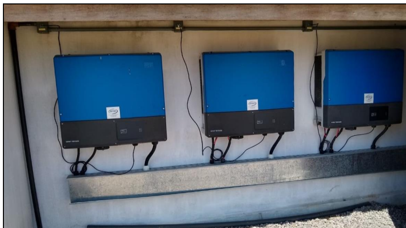
Figura 2 – Inversores SMA Sunny Tripower.
